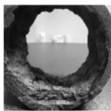
Old cast iron Pipe
